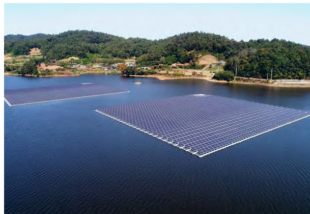
AquaPower installed in Owl Reservoir
